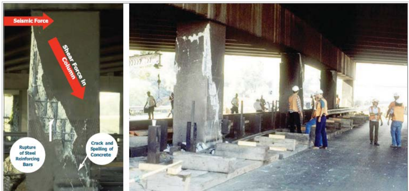
FIGURE 5: Shear Damage of Short Columns at I-5/I-605 Separation
