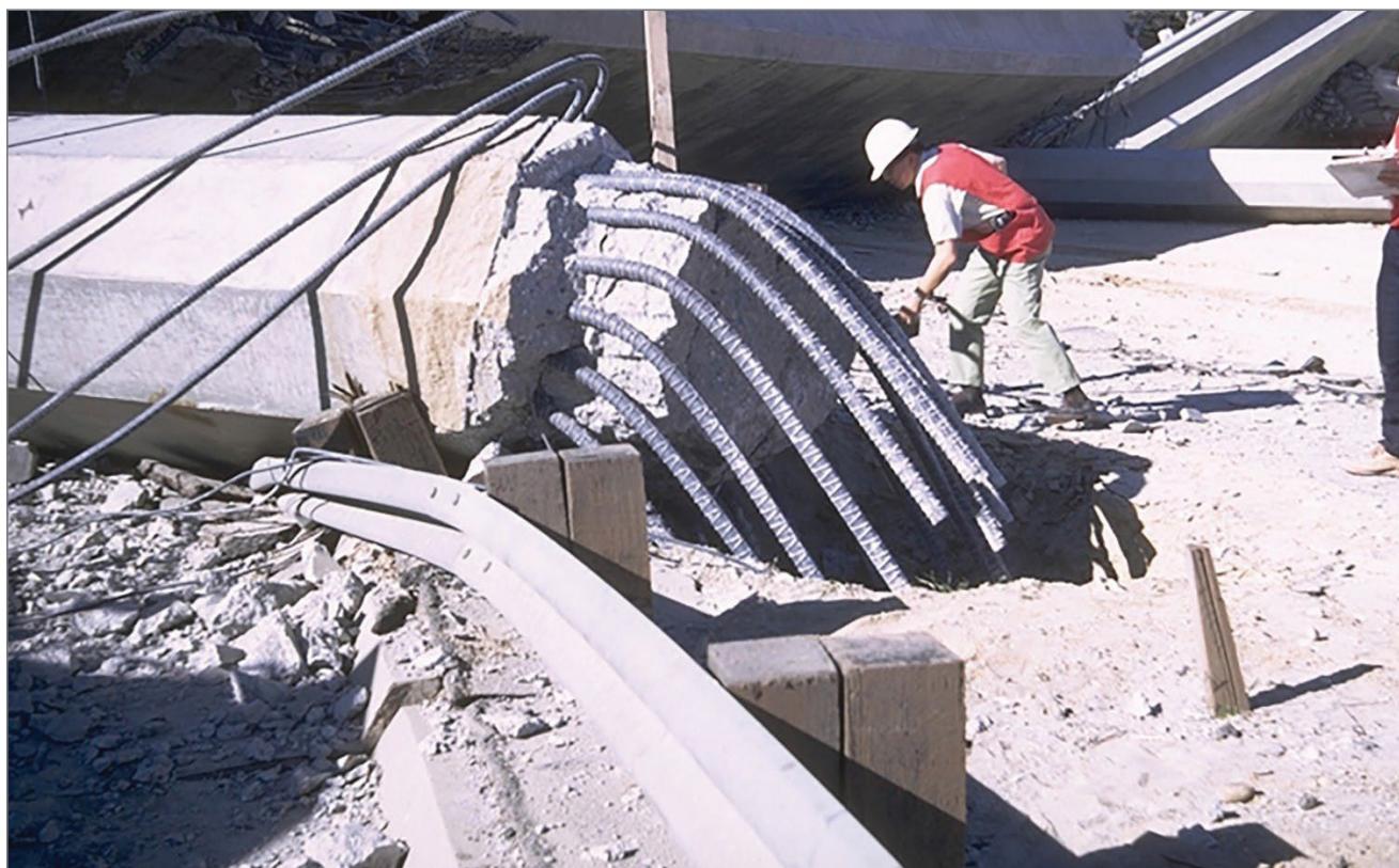
FIGURE 4: Lap Splices at the Column Base Caused Collapse at Route I-210/I-5 Separation and Overhead
