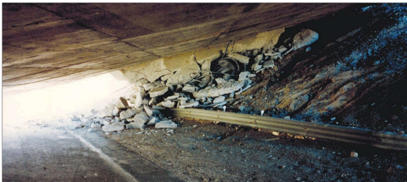
FIGURE 10: Failure of a Short Column at the I-14/I-5 Connector Separation and Overhead
