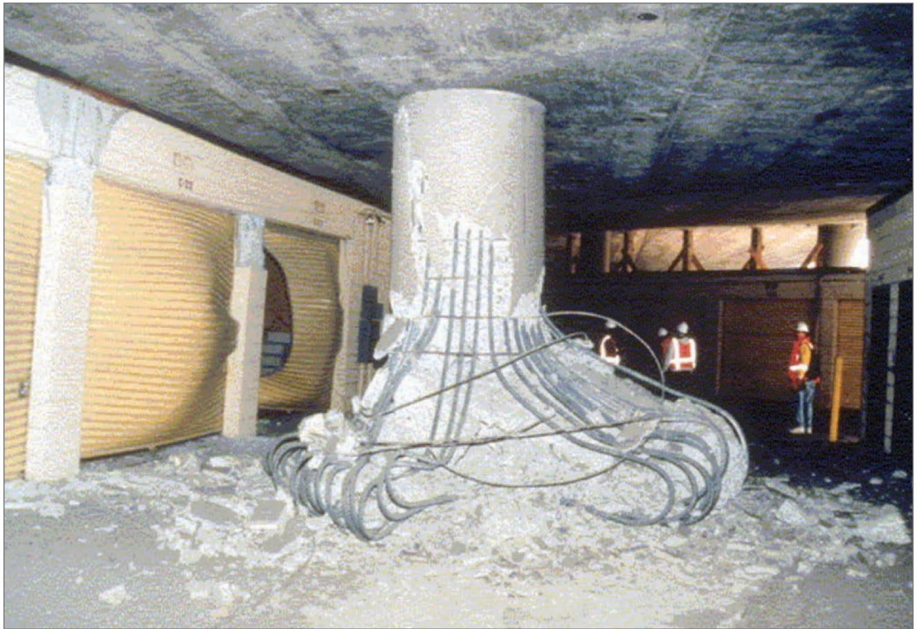
FIGURE 9: Failure of the Santa Monica Viaduct Column
