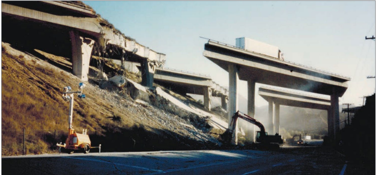
FIGURE 12: Unseated Highly-Skewed Bridge Spans at the Gavin Canyon Bridge
