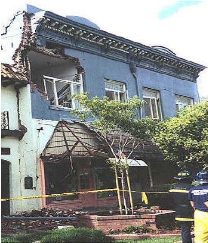
Figure 3.85 – Partial collapse of a brick wall in a historic building in downtown Santa Cruz following the 1989 Loma Prieta Earthquake.
