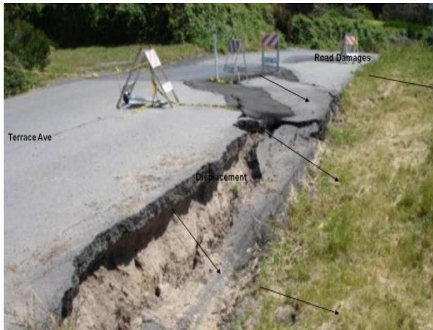
Figure 4.11 – Road damaged by a small landslide scarp. Photo courtesy Cal OES.
