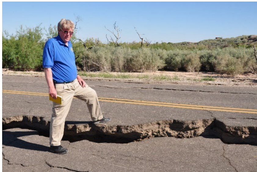
Figure 4.12 – Road damage due to a fault scarp following the 2010 Baja Earthquake. Photo courtesy Fred Turner, EERI.
