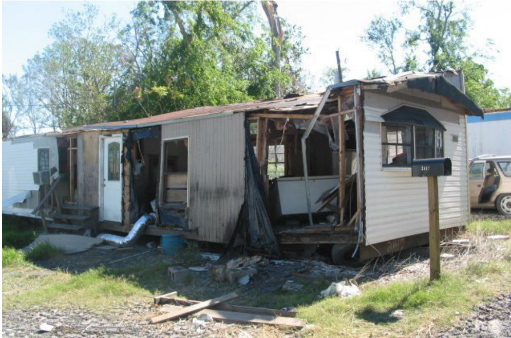
Figure 3.73 – A manufactured home was damaged in 2005 Hurricane Katrina. Photo courtesy Raymond Lui.
