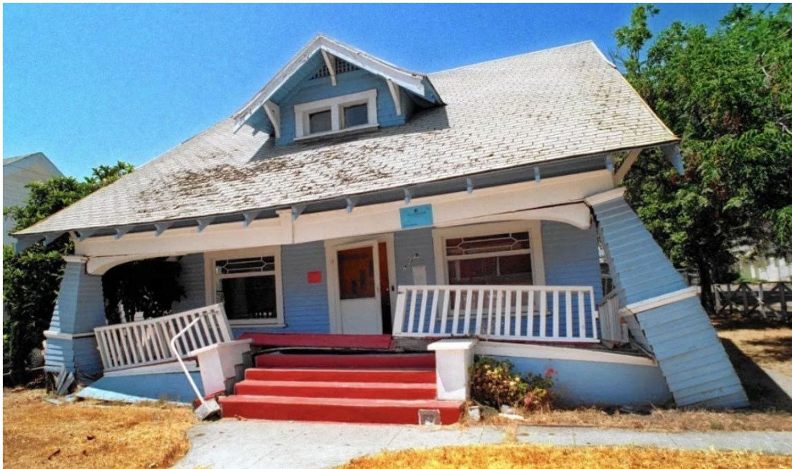
Figure 3.80 – A Craftsman style home suffered heavy damage in an earthquake.
