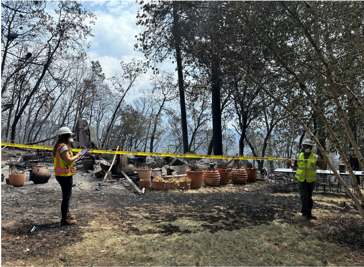
Figure 3.29 – Park Fire 2025. Multiple environmental hazards are present on the property. On the left side, there is a chimney that can be a potential fall hazard. SAP Evaluators place a fall hazard zone around the perimeter.
