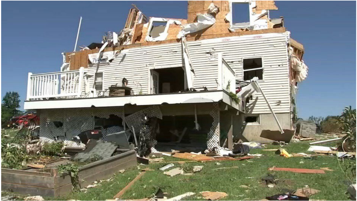
Figure 3.17 – A 2021 tornado in New Jersey heavily damaged this house.
