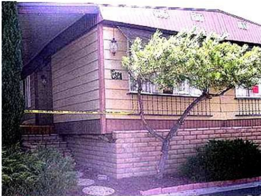
Figure 3.74 – This manufactured home was damaged in an earthquake. The steel frame shifted and is shown resting on the decorative but fragile brick skirting. The marriage line of this double-wide seems to be ready to pull apart at the bottom. Home was tagged UNSAFE and barricaded with caution tape.
