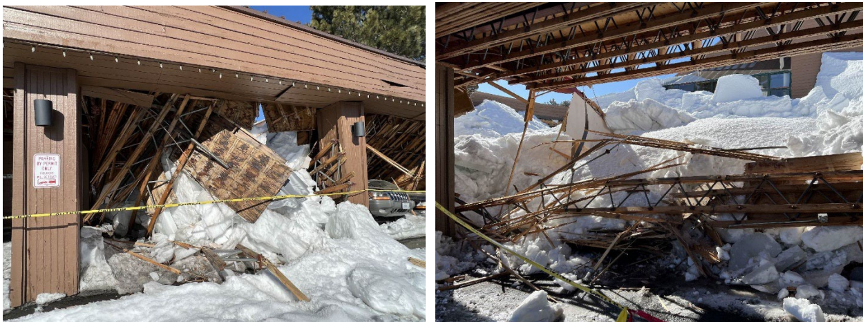
Figure 3.60 – Complete collapse of overhead structure due to snow load. 2023 Mono County Snow Load Mission. Photos courtesy Gurbir Singh.
