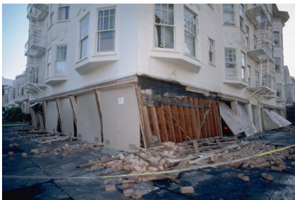
Figure 3.5 – Partial soft story failure, 1989 Loma Prieta Earthquake.
