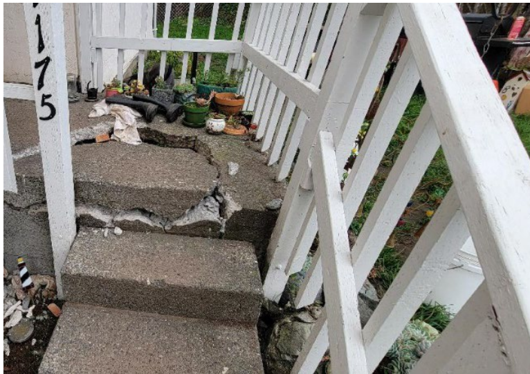
Figure 3.44 – Wood beam across front porch cracked due to snow load. House was tagged RESTRICTED USE to prevent use of front door. 2023 Mono County Snow Load Mission. Photo courtesy Gurbir Singh.
