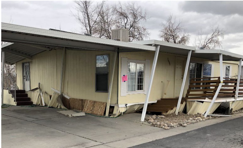
Figure 3.70 – Manufactured home damaged in an earthquake. Collapsed on foundation piers. Tagged UNSAFE.
