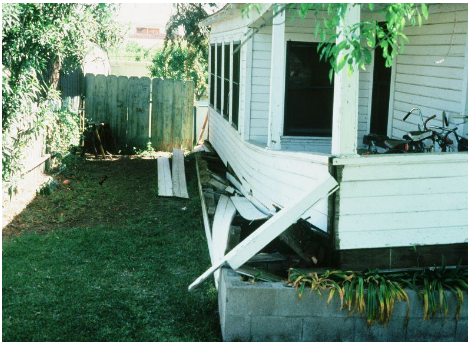
Figure 3.9 – House slid off its foundation, 1994 Northridge Earthquake.
