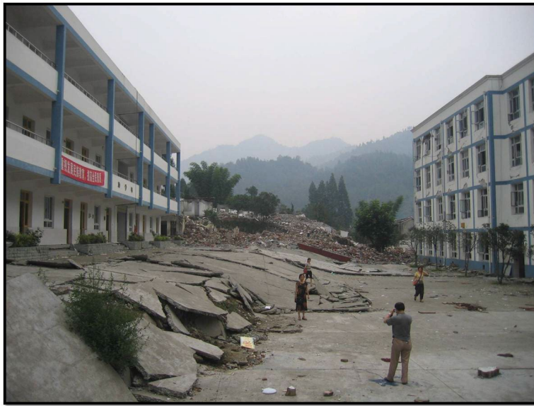
Figure 4.3 – Fault scarp developed between two apartment buildings in Taiwan.
