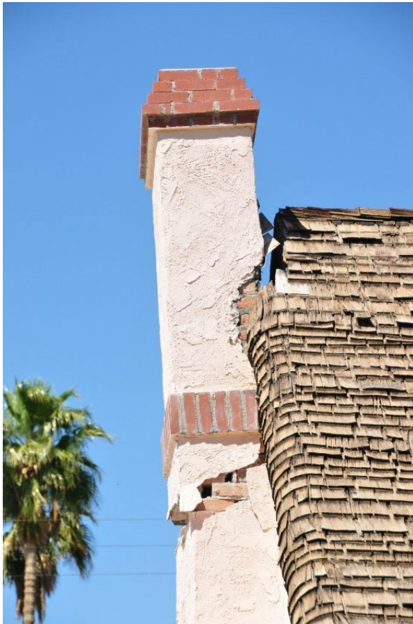
Figure 3.7 – Cracked chimney, 1994 Northridge Earthquake.
