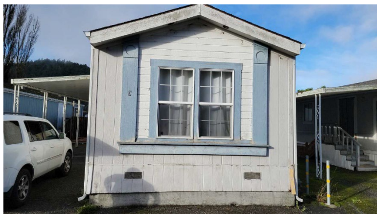
Figure 3.41 – Manufactured home survived 2022 Ferndale Earthquake. Shifted one inch on its foundation. Tagged INSPECTED. Photo courtesy Gurbir Singh.
