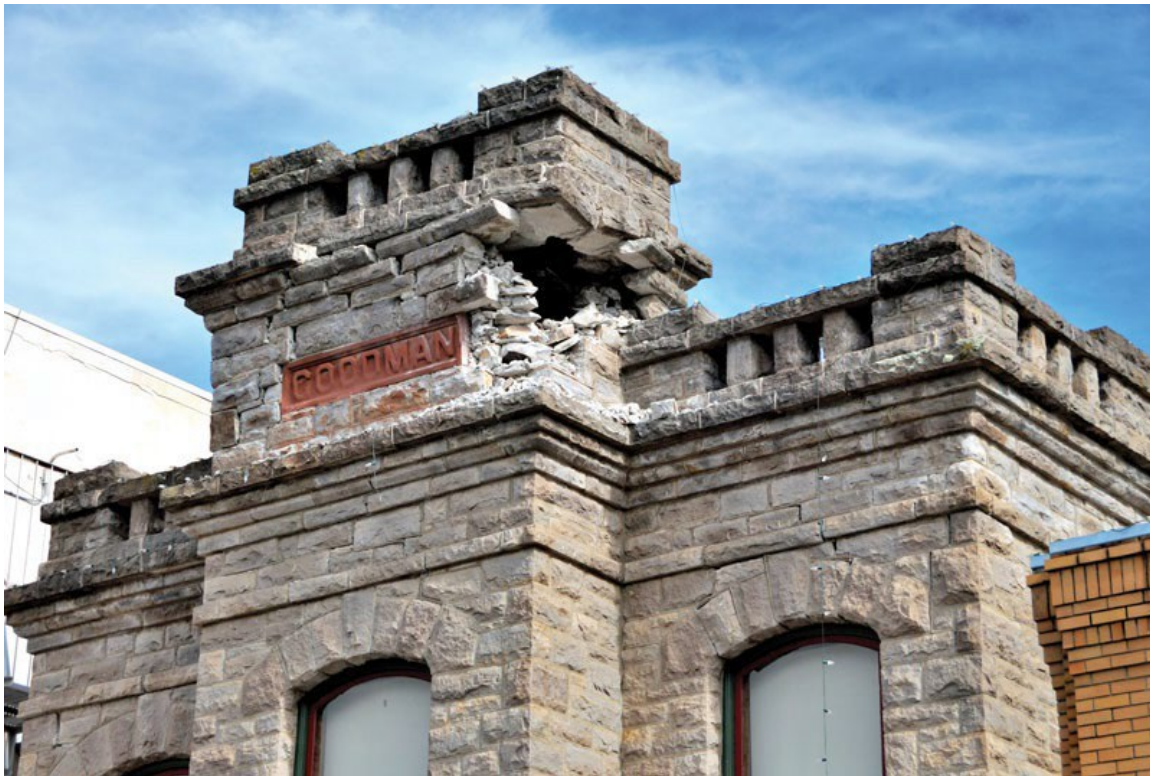
Figure 3.82 – Damage to the Goodman Library Building in Napa due to the 2014 Napa Earthquake.
