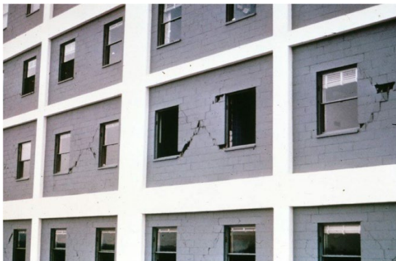
Figure 3.4 – Shear cracking in masonry infill wall.
