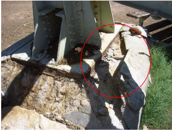
Figure 3.50 – Base plate movement at the El Centro Water Tower spalled the grout on the footing. Photo courtesy David Karina.
