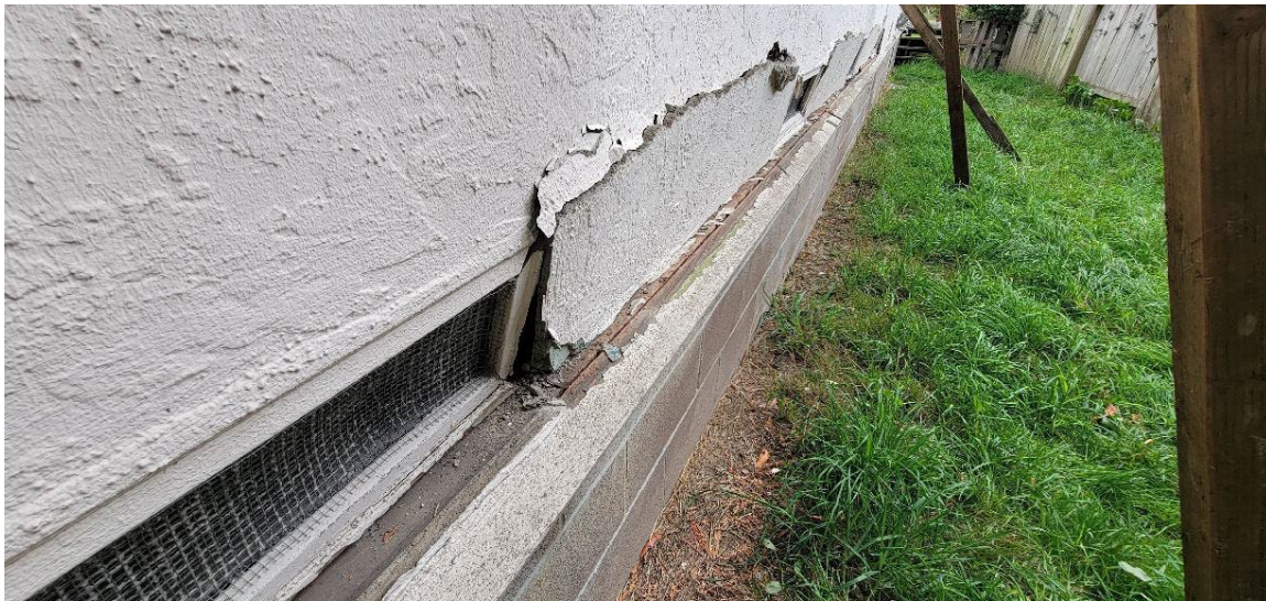
Figures 3.43 – House survived the 2022 Ferndale Earthquake. Damage to the front entrance stairs, damage to stucco and interior plaster, but the structure is still livable. Tagged INSPECTED. Photos courtesy Gurbir Singh.
