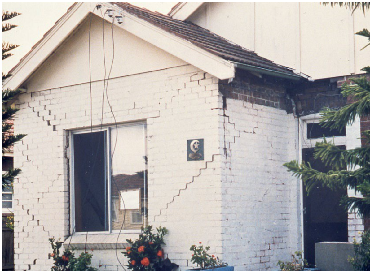
Figure 3.69 – Example of shear cracking in masonry wall house.
