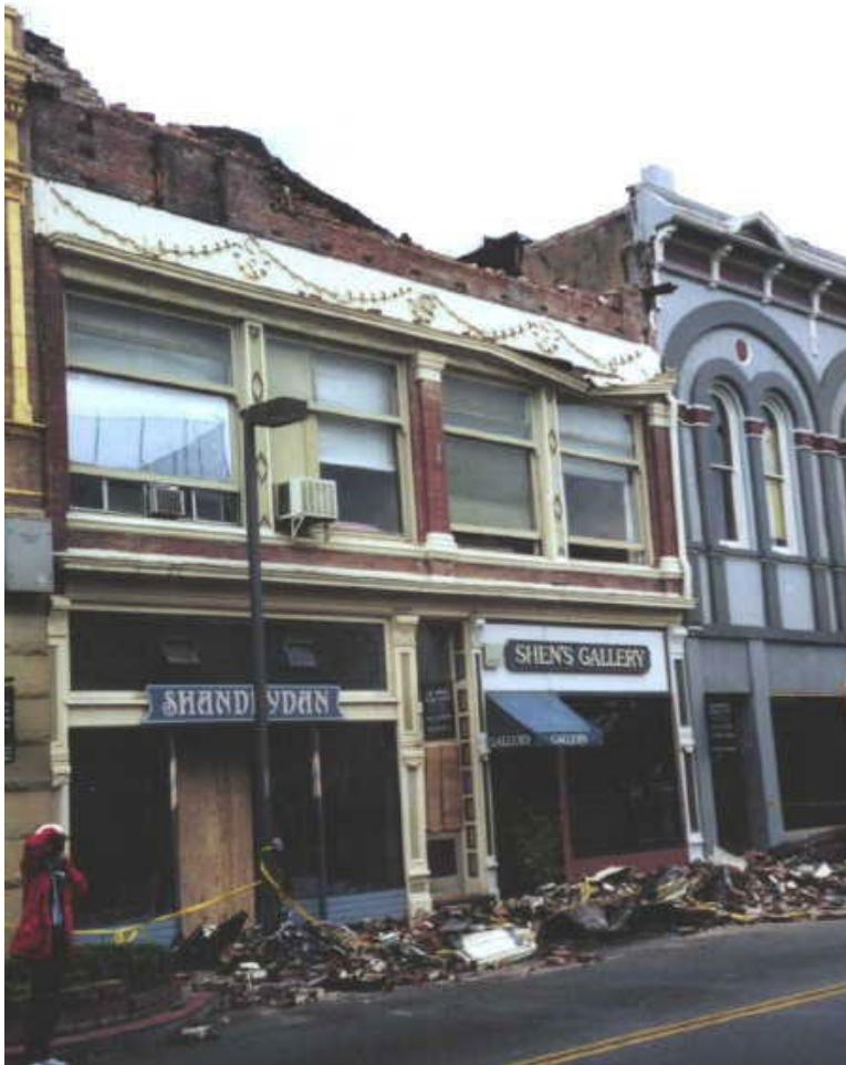
Figure 3.84 – Parapet failure in a historic building in downtown Santa Cruz, due to the 1989 Loma Prieta Earthquake.
