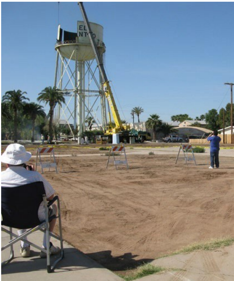
Figure 3.52 – The collapse hazard caused by the El Centro Water Tower was abated by demolition. Photo courtesy David Karina.
