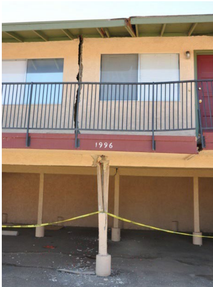
Figure 4.22 – Large crack between rigid and failed parts of upper story. Photo courtesy Fred Turner, EERI.
