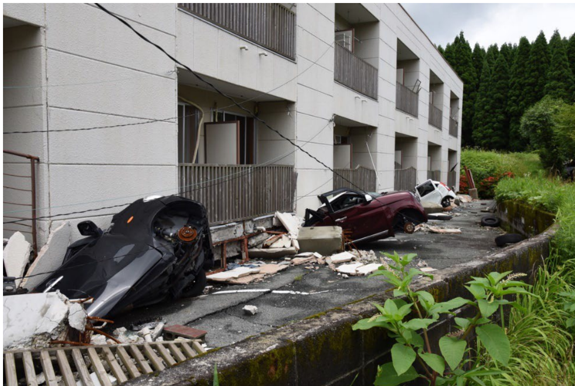
Figure 3.67 – Full collapse of soft story. Apartment building completely crushed the parking floor underneath it, including cars.
