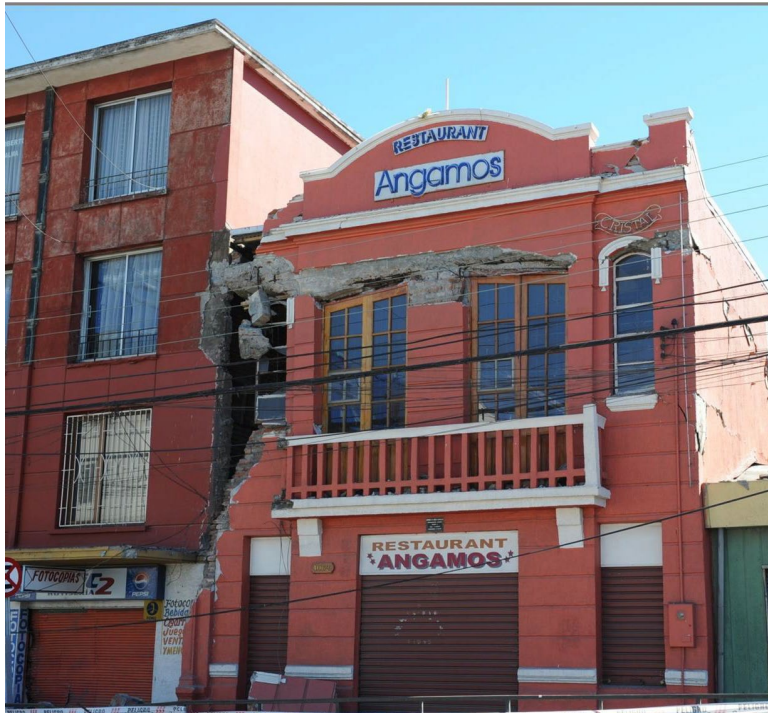
Figure 3.6 – Effects of seismic pounding, Chile.
