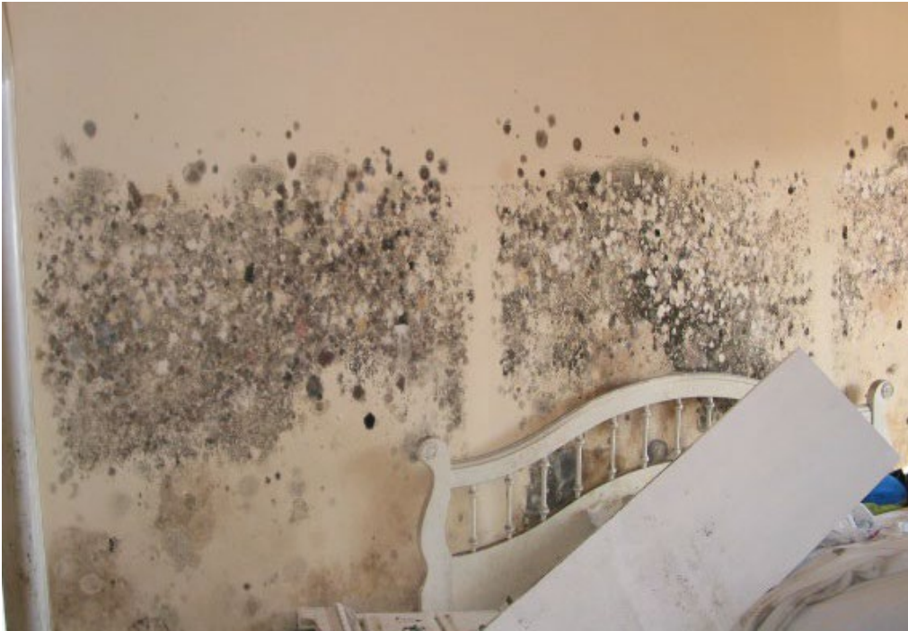
Figure 5.16 – Mold infestation following a flood disaster. Photo courtesy Raymond Lui, SEA.
