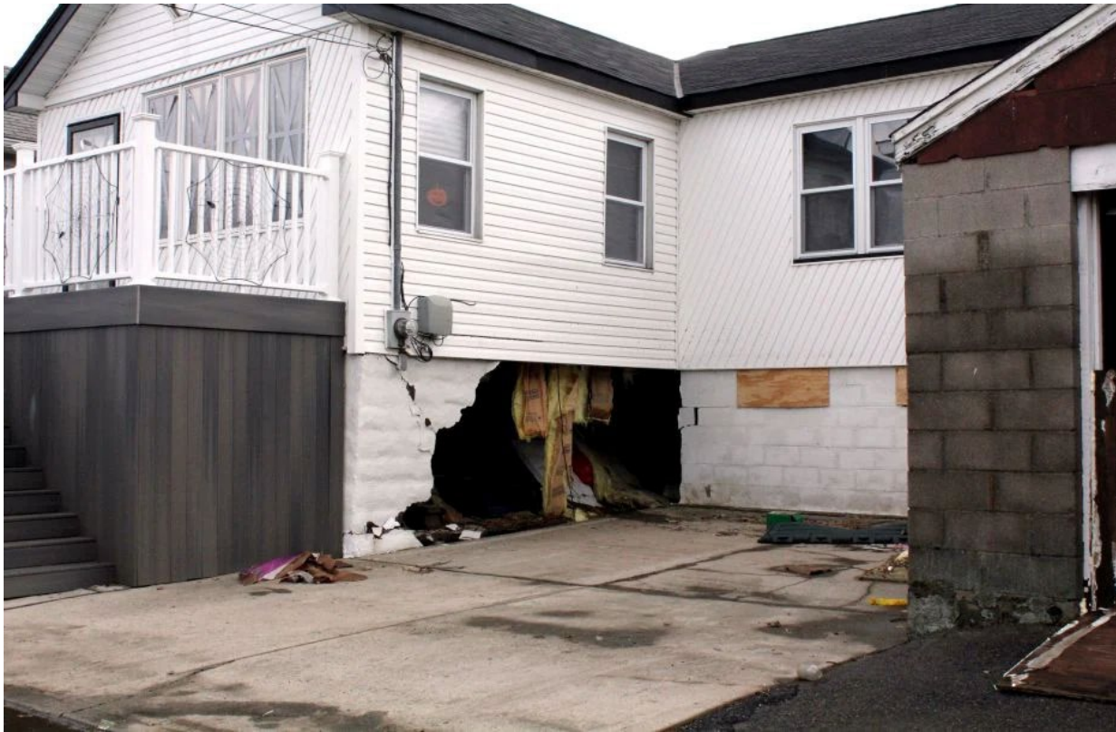
Figure 3.12 – Flood damage to foundation wall, 2012 Hurricane Sandy.
