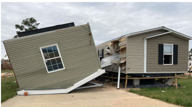
Figure 3.72 – A double-wide manufactured home split apart in a hurricane and a section rolled over.
