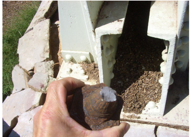
Figure 3.51 – Excessive movement in the structure of the El Centro Water Tower caused rivets to pop. Photo courtesy David Karina.
