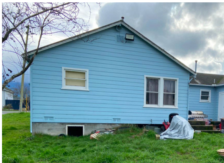
Figure 3.42 – House survived the 2023 Ferndale Earthquake. Minor drywall cracks and a minor crack in concrete foundation observed; could have been present before the earthquake. Tagged INSPECTED. Photo courtesy Gurbir Singh.
