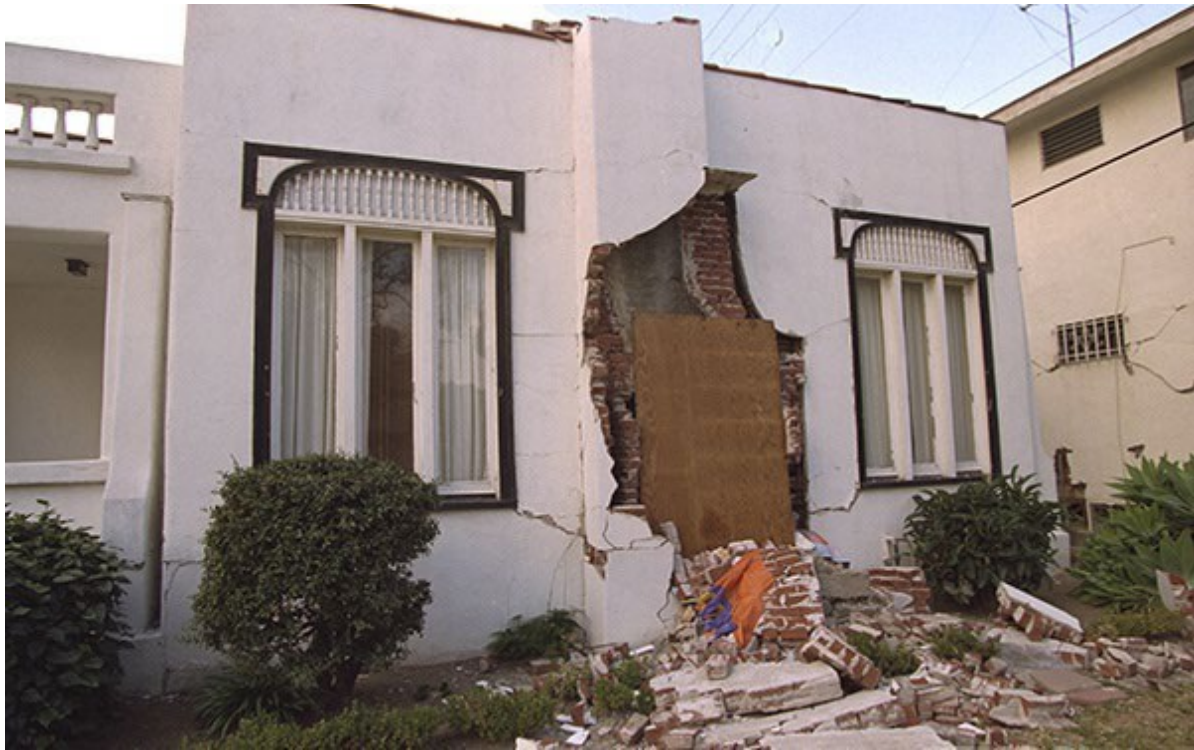
Figure 3.68 – Earthquake destroyed chimney.
