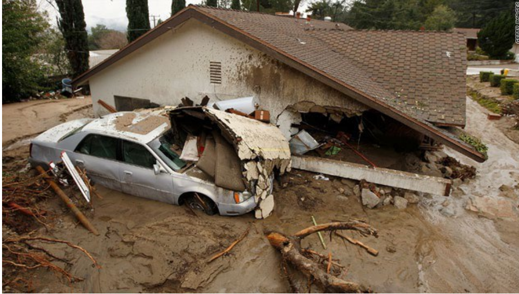
Figure 3.37 – Mudflows damage a home in La Canada Flintridge in 2010.
