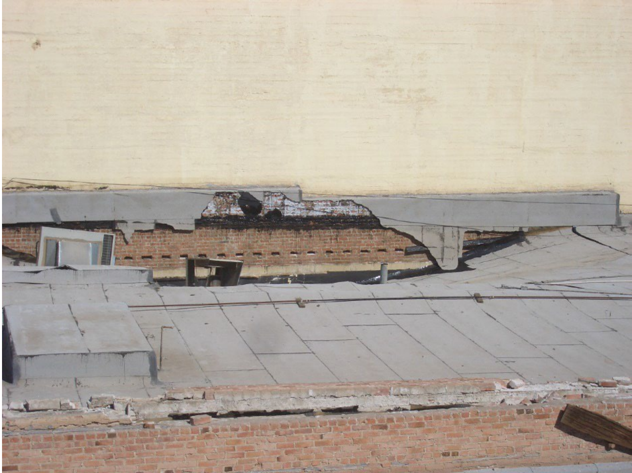
Figure 3.65 – Roof diaphragm pulled out from supports in brick wall during the 2010 Baja Earthquake. Photo courtesy David Karina.
