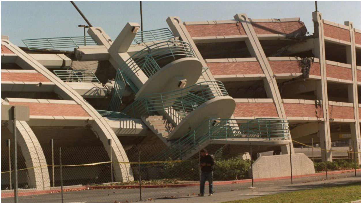
Figure 3.64 – Failed parking structure from the 1994 Northridge Earthquake.
