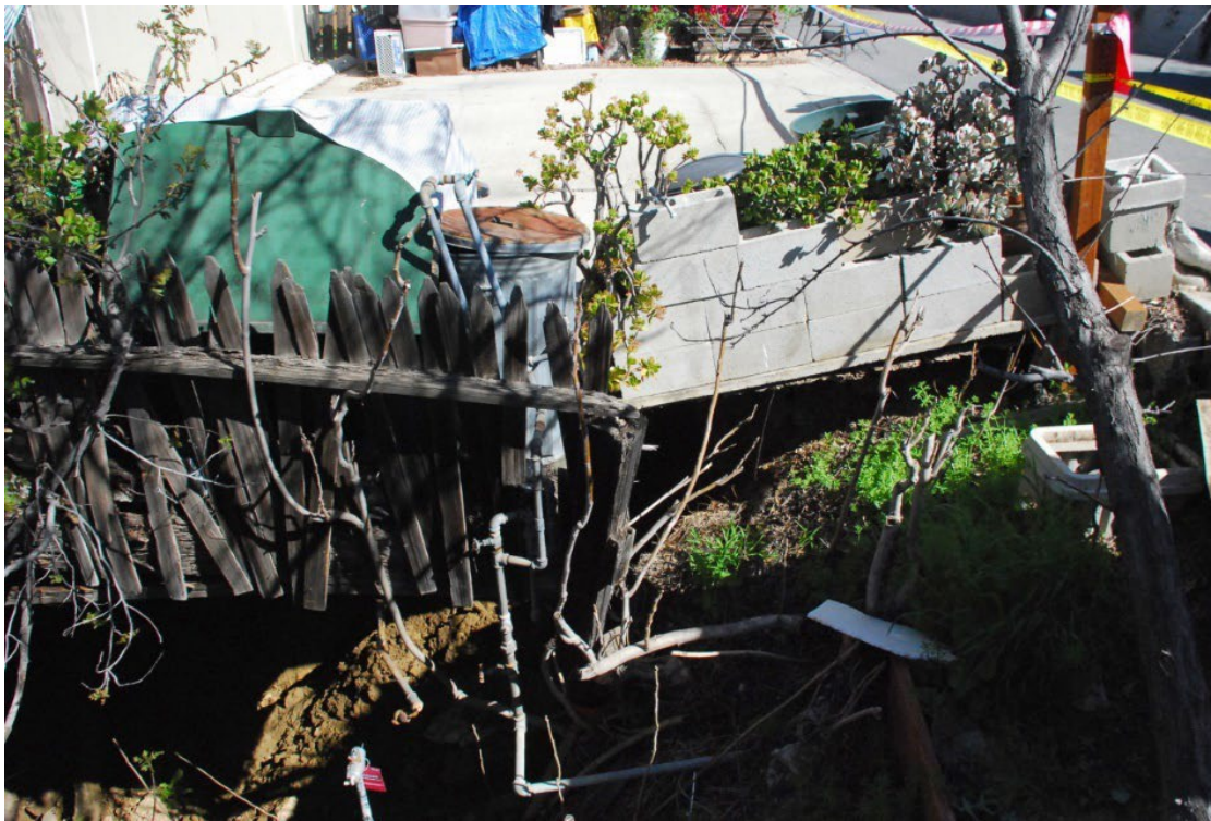
Figure 3.62 – Home in South Pasadena was undermined by a broken water main, was evacuated due to threat of imminent structural failure.
