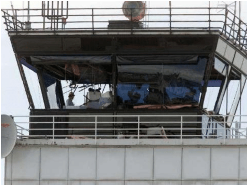
Figure 4.6 – Damaged aircraft control tower.
