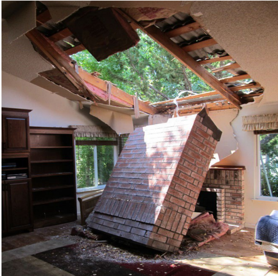
Figure 3.8 – Collapsed chimney through roof, 2014 Napa Earthquake.
