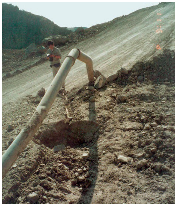
Figure 4.14 – Pipe damaged by faulting in the 1990 Manjil Earthquake in Iran.
