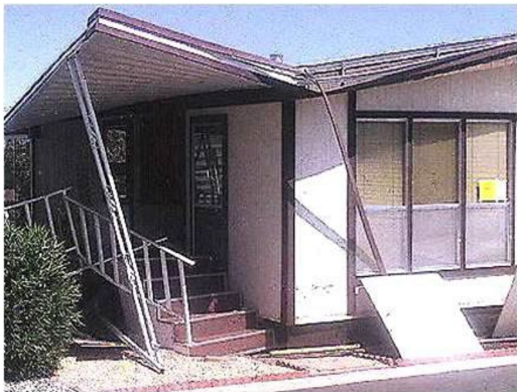
Figure 3.76 – Manufactured home collapsed on its supports. Stairs are now partway up in the door, and the side awning is unstable. Was tagged RESTRICTED USE, likely for possession retrieval.
