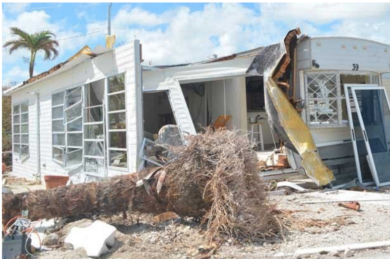
Figure 3.71 – Manufactured home damaged in a hurricane.
