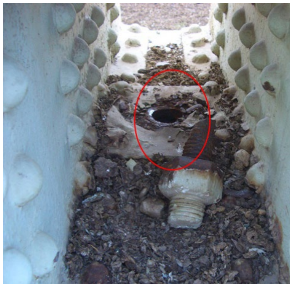
Figure 3.49 – Bolt at pad footing of the El Centro Water Tower was sheared off due to earthquake. Photo courtesy David Karina.
