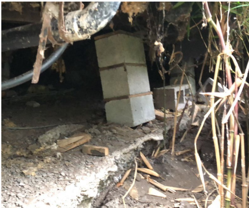
Figure 3.61 – Manufactured home shifted and twisted 4 inches off its foundation piers, which were rendered unstable. 2022 Ferndale Earthquake. Photos courtesy Gurbir Singh.
