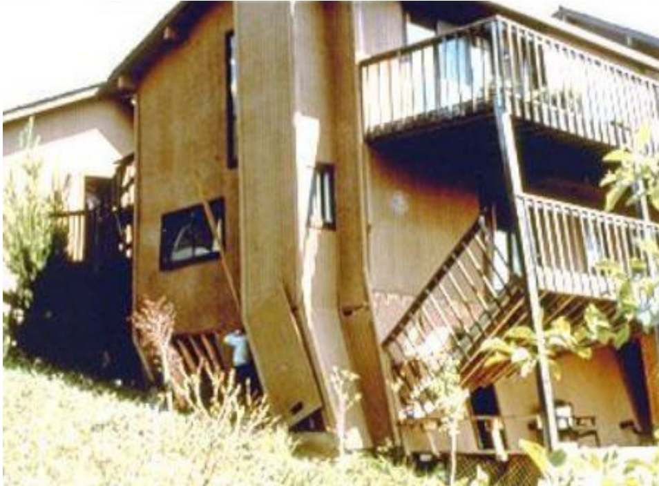
Figure 3.87 – Soft story damage to apartment building on hillside from the 1984 Morgan Hill Earthquake. Note the man entering the structurally compromised understory area of this building; do not do this! Also, stepping onto the second story porch could be dangerous; it might be simply leaning against the building, rather than attached to it, considering that the first story porch is no longer attached.
