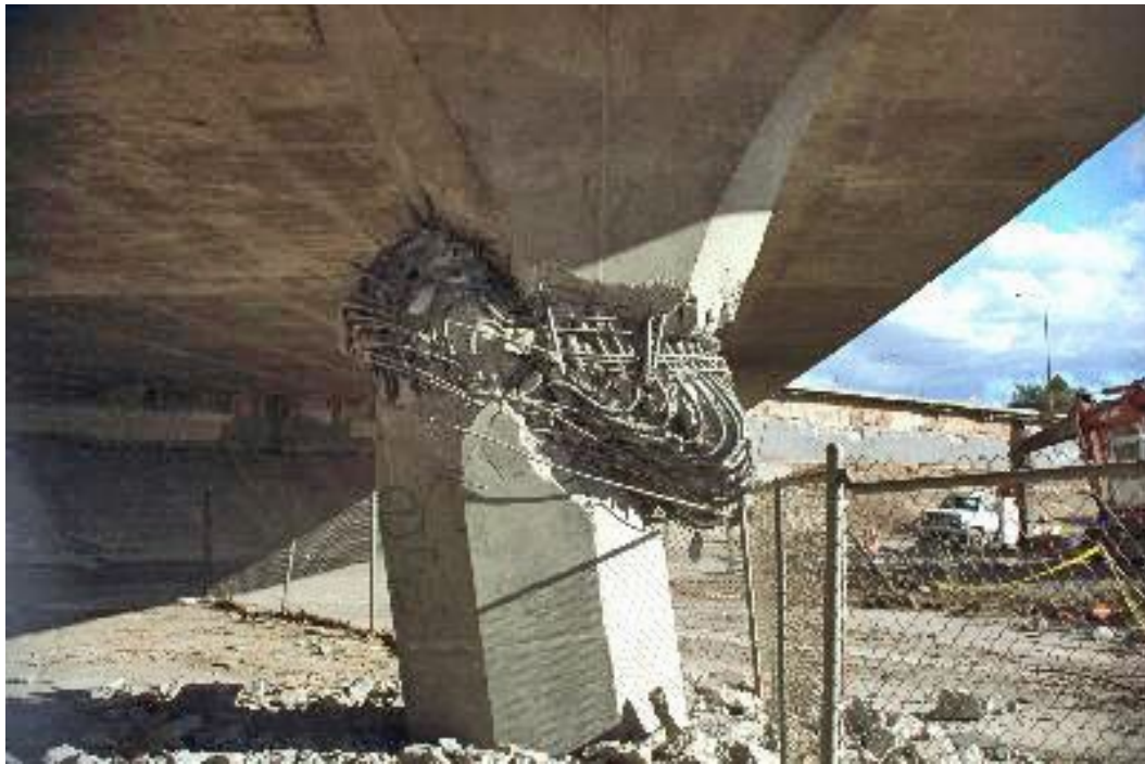
Figure 4.9 – Interstate 10 column collapse, 1994 Northridge Earthquake.
