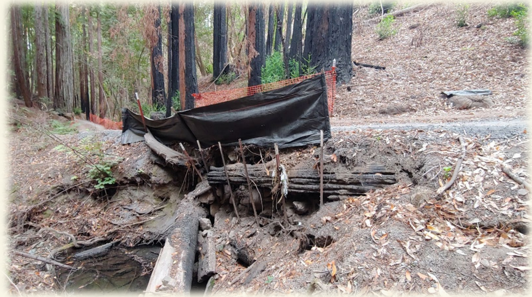
Humboldt Crossing fire damage – access point to parcel
