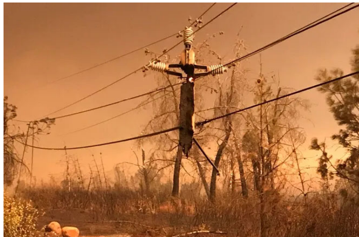
Remnants of a telephone pole hang from their lines after they burned in Camp Fire on Thursday, Nov. 8, 2018. Photo Credit: Jim Schultz
