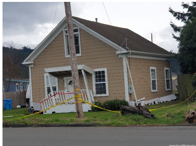
Damaged home in Humboldt County. Source: Clearinghouse/EERI
