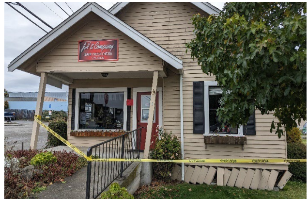
Red-tagged local business in Humboldt County. Source: Clearinghouse/EERI
