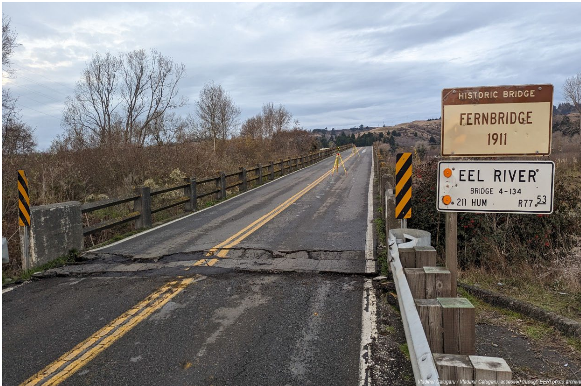
Photo of Fernbridge damage in Humboldt County. Source: Clearinghouse/EERI
