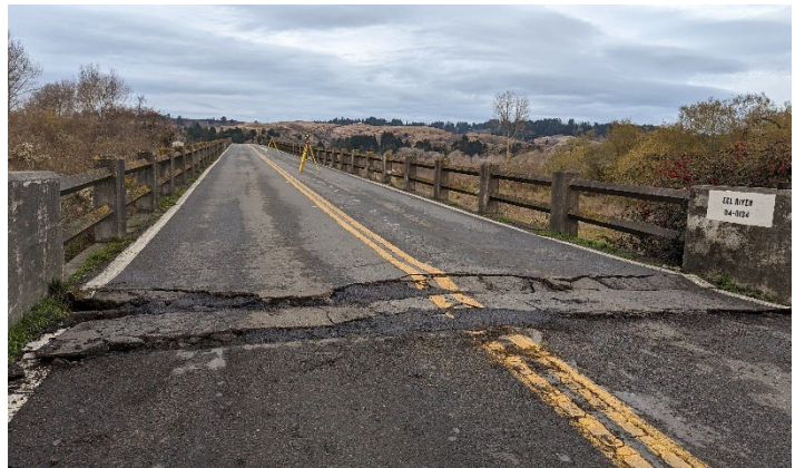
Road damage due to M6.4 earthquake in Humboldt county. Source: Clearinghouse/EERI
