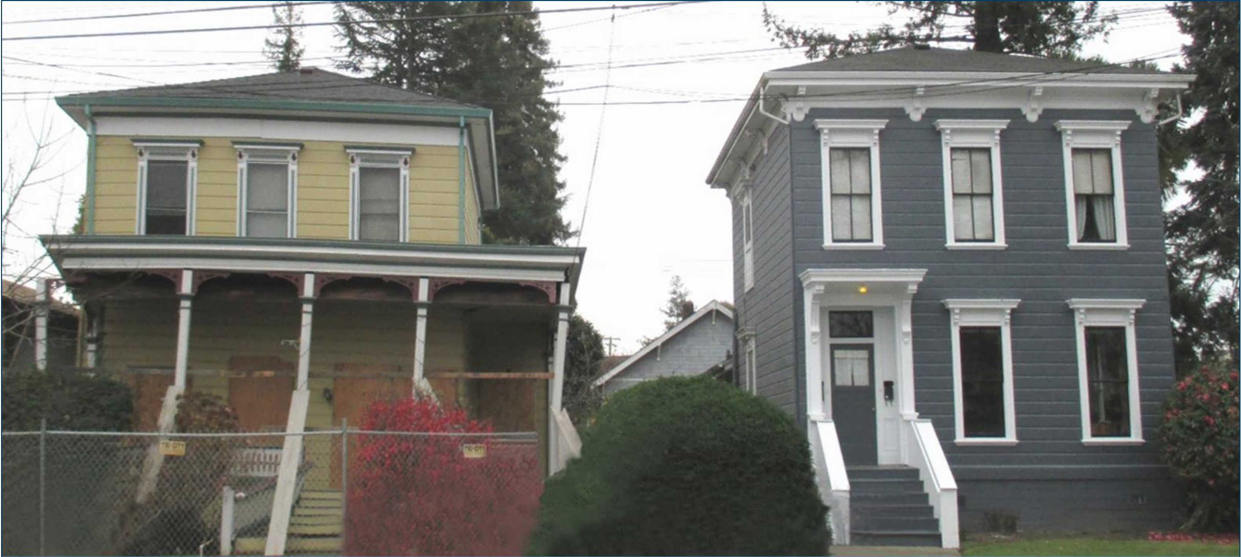
Unretrofitted – Red Tagged
