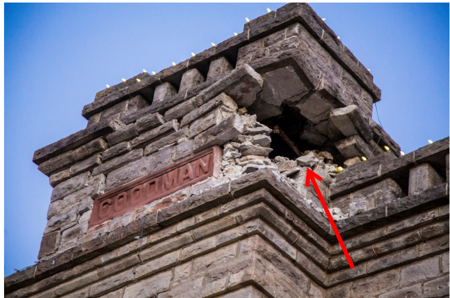
The top of the Goodman Library's façade was damaged by the August 24, 2014 earthquake. (Photo: Christopher Mardorf)
