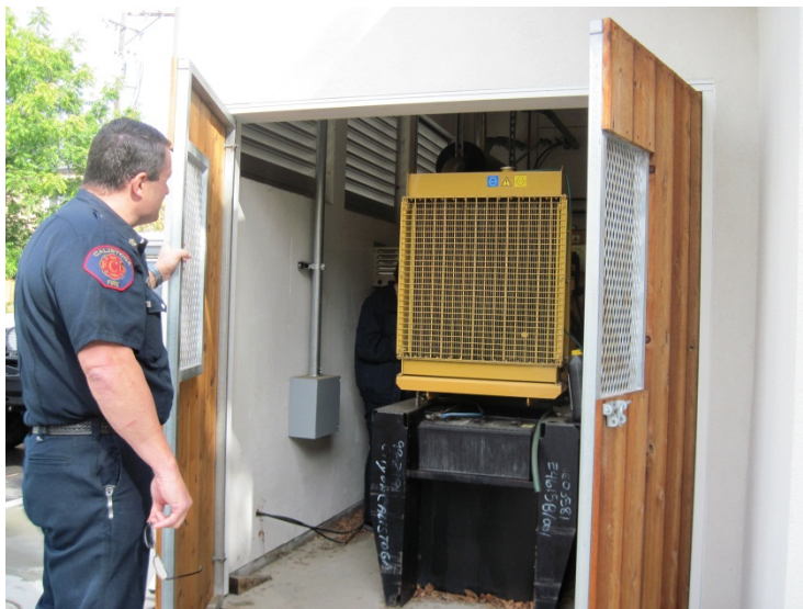
Chief Campbell shows off the emergency generator and its 200-gallon fuel tank which are bolted down and the generator wiring which is strapped to the wall. (Photo: Bonnie Hanchett)
