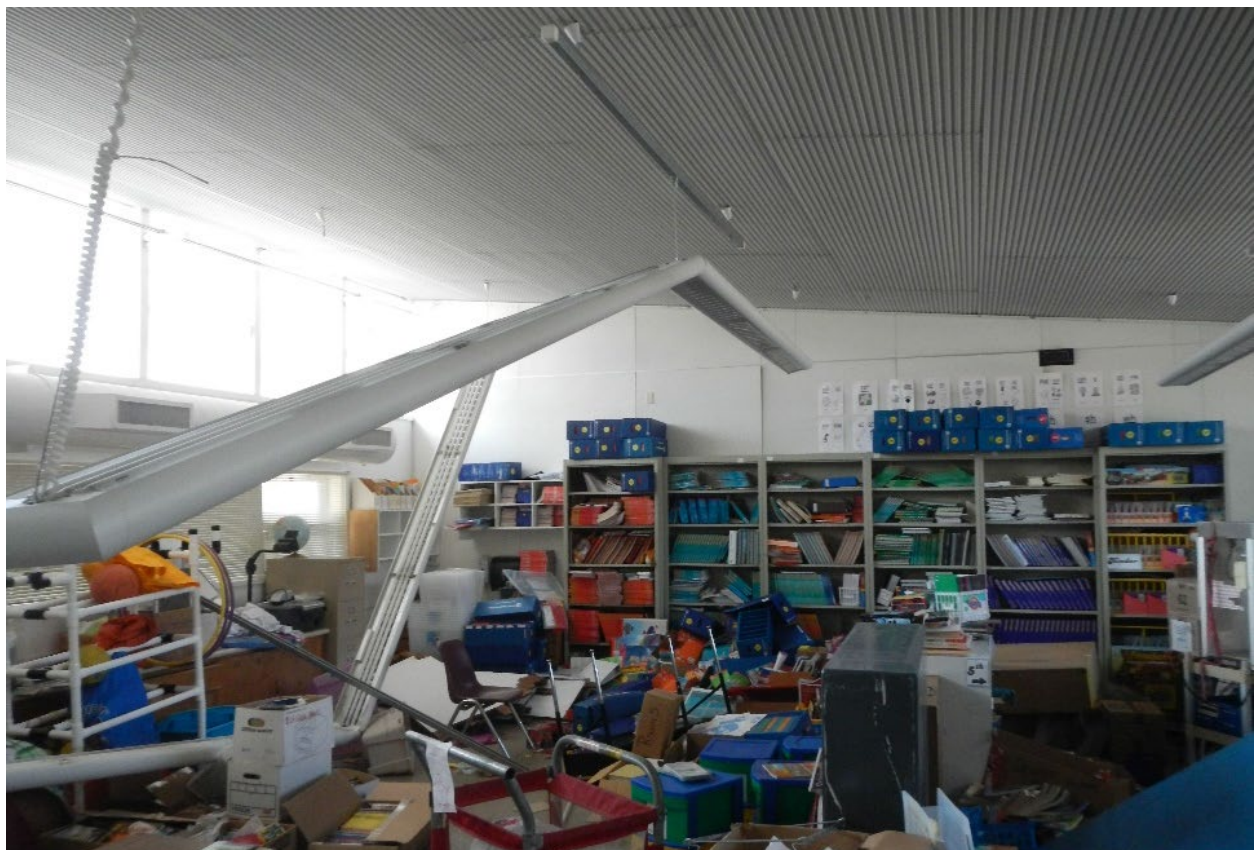
2014 South Napa Earthquake damage to Napa Valley Unified School District, California (from M. Quattrocchi).
