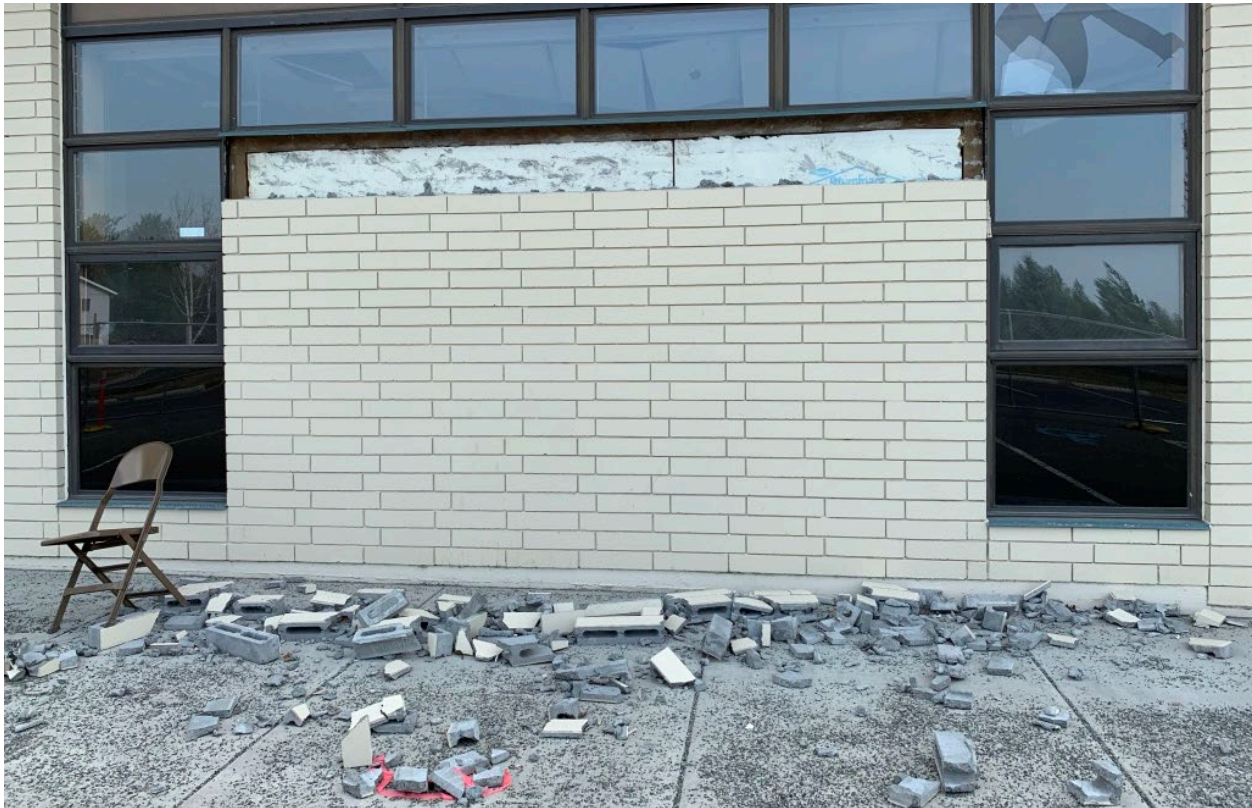
2018 Anchorage Earthquake damage to Anchorage School District, Alaska (from the Earthquake Engineering Research Institute).
