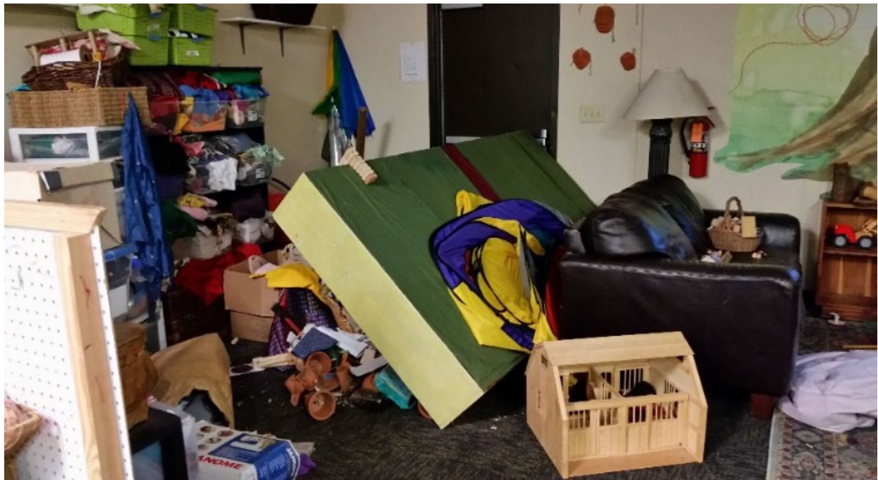
2018 Anchorage Earthquake damage to Matanuska-Susitna Borough School District, Alaska (from Earthquake Engineering Research Institute).
