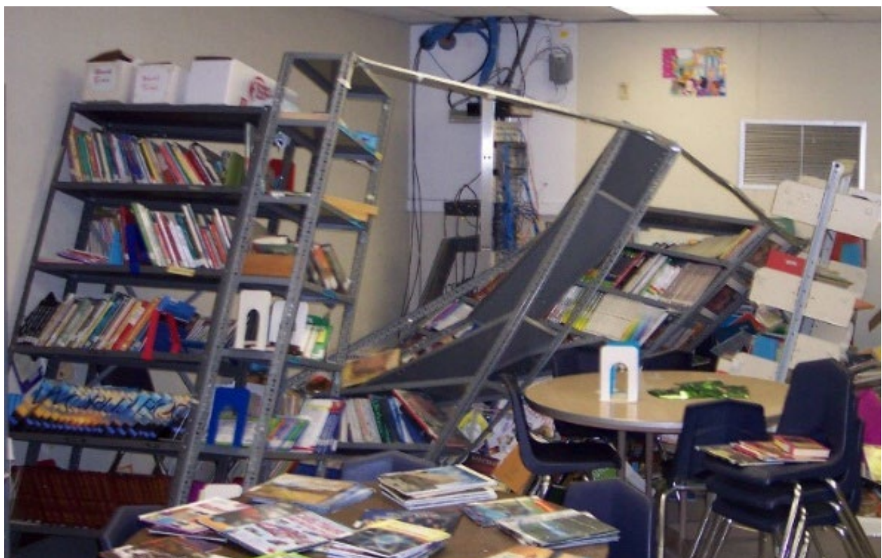
2010 Mexicali Earthquake damage to Calexico Unified School District, California (from California Division of the State Architect).
