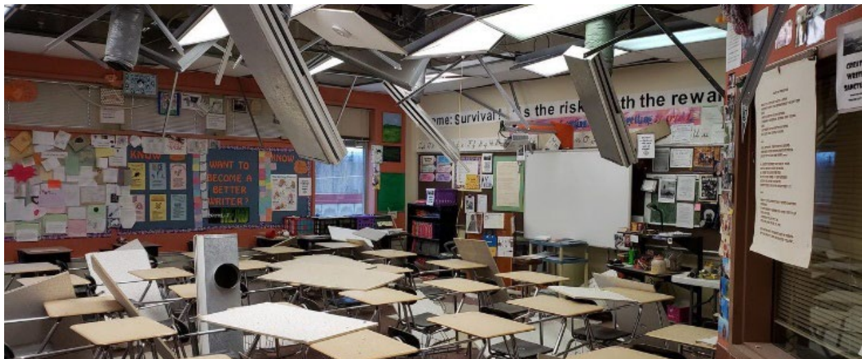
2018 Anchorage Earthquake damage to Matanuska-Susitna Borough School District, Alaska (from Earthquake Engineering Research Institute)
