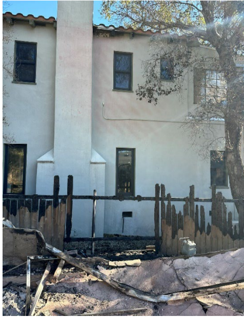
Figure 21. The fence that was attached to the home ignited, causing fire spread to the home.
