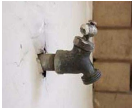
Figure 23. The gap around utility penetrations such as this one should be sealed with a fire-resistant material.
